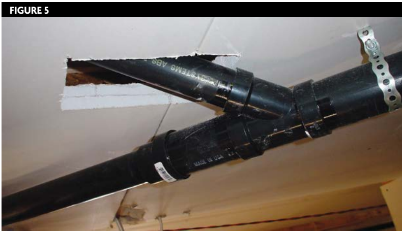
Example of combustible pipe penetration at an angle. No tested firestop systems exist in this situation.
