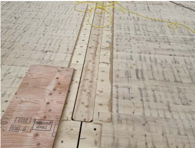
Wood cover over isolation pad. PHOTO COURTESY AERCOUSTICS ENGINEERING LIMITED
