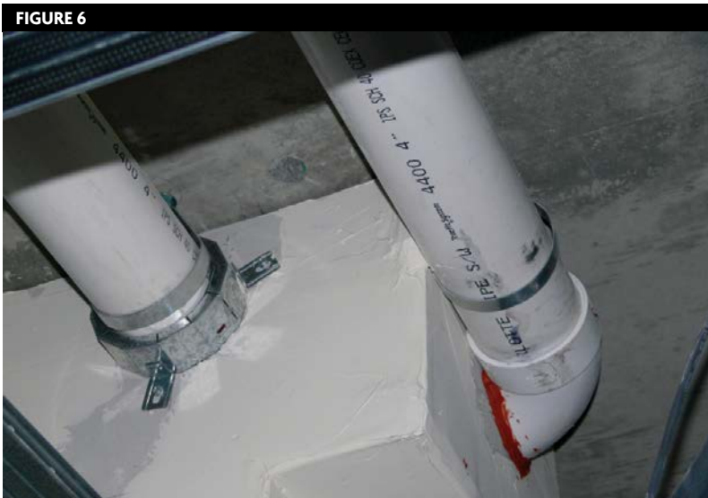
Examples of penetrations with available firestop listings (perpendicular, unobstructed) and without available firestop listings (no room for intumescent collar).
