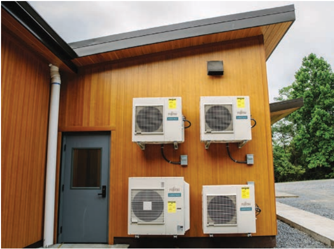
Existing forced air systems in large buildings can now be retrofitted with inverter heat pumps, thanks to direct exchange (DX) kits, which permit the use of custom refrigerant coils in large, old air handlers.
