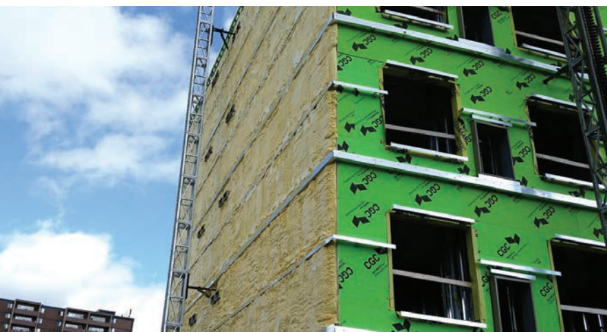
With batt insulation and polyethylene located on the interior side of the assembly, the architect sought an exterior insulation system that would allow for outward drying.
