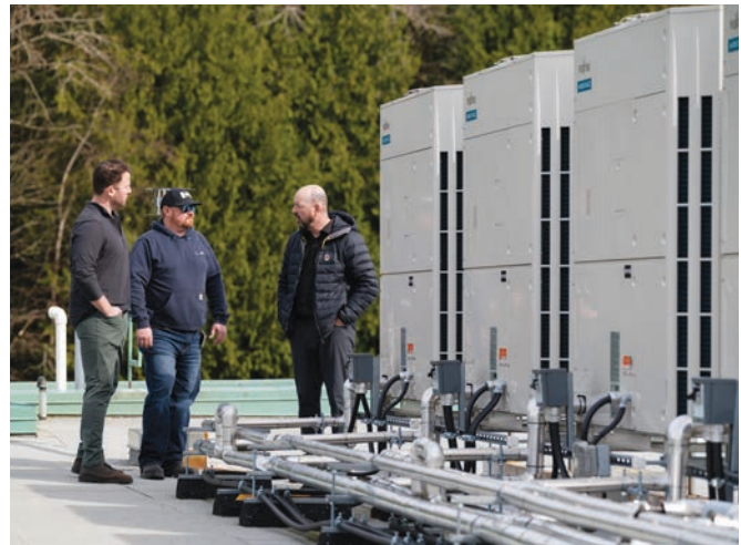
Variable refrigerant flow (VRF) systems installed at an elementary school in British Columbia.
