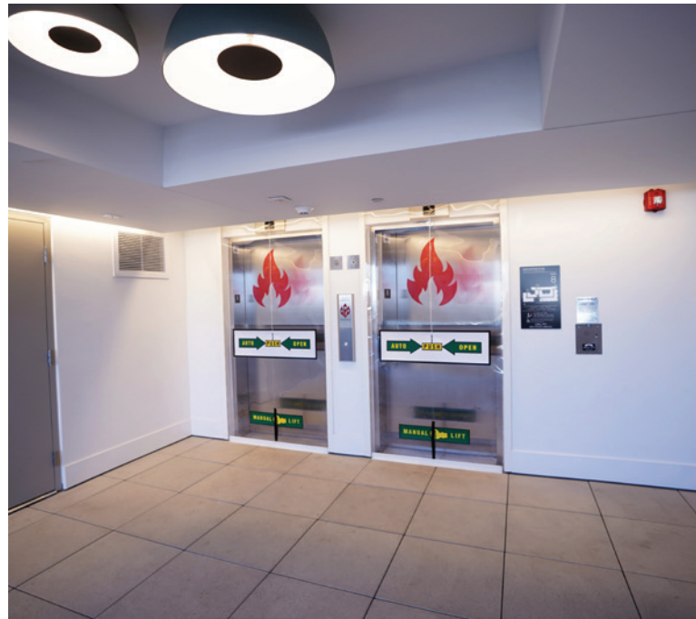
Seal openings on elevators in this data centre block smoke spread in multi-floor data centres, maintaining clear paths for occupants and first responders.
