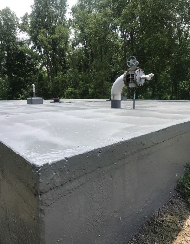
Water tank application.
